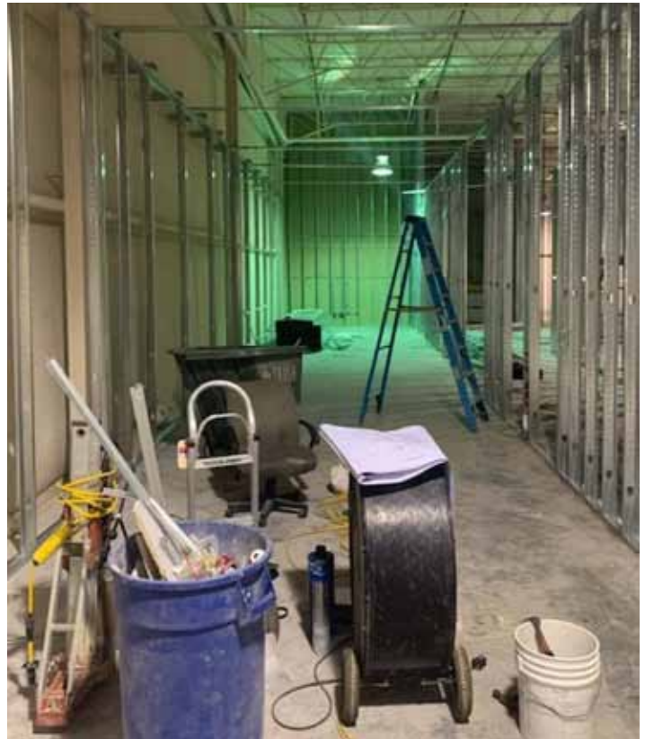
UNDER CONSTRUCTION: Work is underway inside NRVCS' Radford Center to establish a new home for the New Horizons crisis stabilization program, which is currently located in Fairlawn. The new site is located adjacent to the Crisis Center and will also allow for increased service capacity. (Photo - R. Burton/NRVCS)
